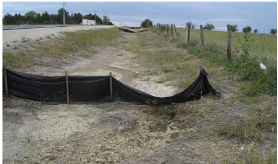
A damaged BMP like this one—a sediment fence wash-under failure in a right-of-way ditch—should be reported to the job site supervisor, and quickly repaired.
