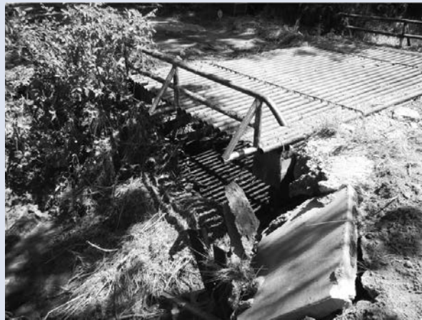
An example of the flood damage: This washed-out entrance was the only entrance into a farmstead. John Remmert, R&B dispatcher, had the field crews take geo-tagged photographs of each site. The sites were mapped using Google Earth.
