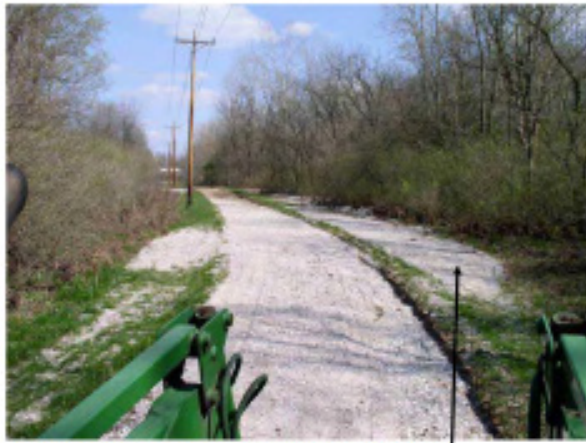
Gravel build-up in natural areas after flooding.
