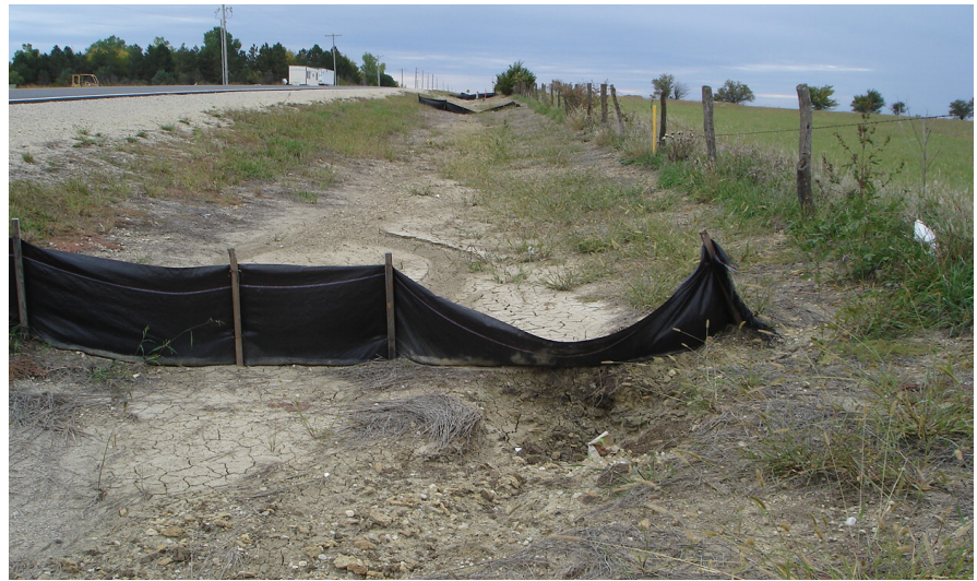
A damaged BMP like this one—a sediment fence wash-under failure in a right-of-way ditch—should be reported to the job site supervisor, and quickly repaired.
